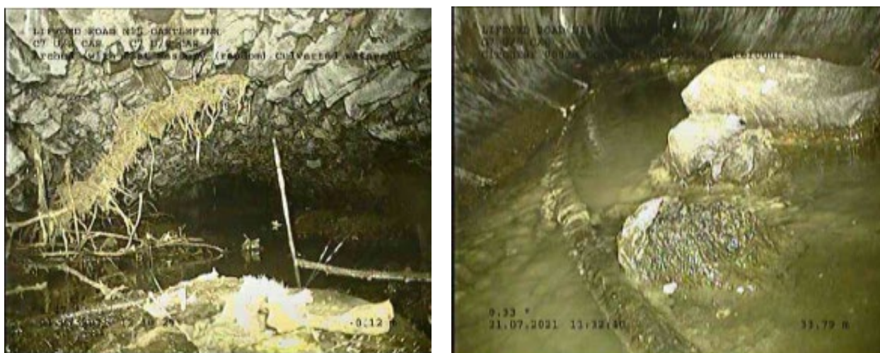
Figure 3.26: (L) Blocked outlet of culvert submerged in water (40% blockage). (R) Internal blockage of culvert
