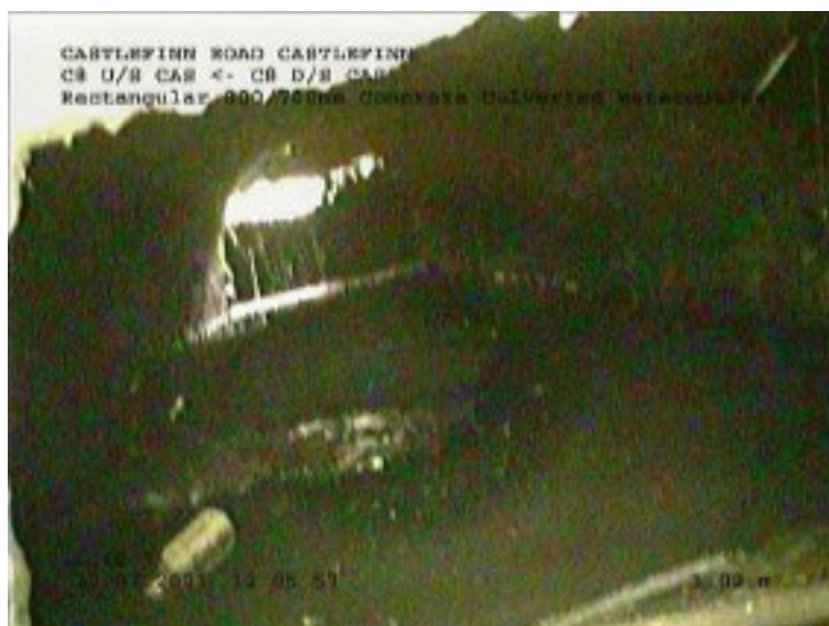
Figure 3.30: Blocked internal conditions of culvert and blockage of debris screen at upstream extent.
