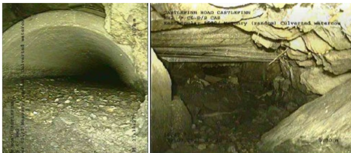
Figure 3.24: (L) Heavily blocked section of McGlynns culverts (90% blockage). (R) View of culvert from manhole chamber.
